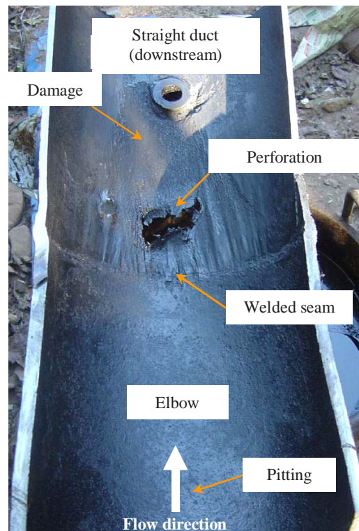
Figure 2. Typical failure downstream of a 90° elbow of a secondary line (Bilmes and Solari, 2008).
