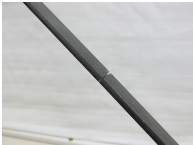
Figure 5: Crack in the strip
